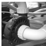
Flanges of the massage pumps
