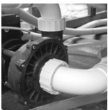
Flanges of the massage pumps
